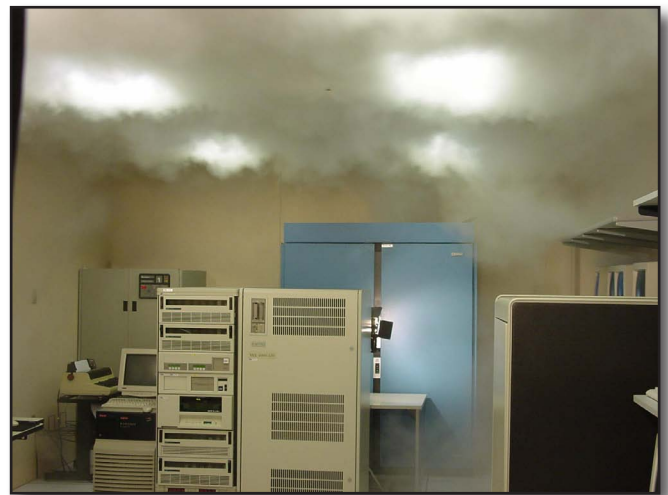
Figure 11-47 Halon Extinguishing System
