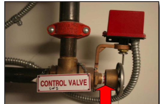
Figure 11-44 Zone/Floor Control Valve Located on Main Riser in Stairwell
