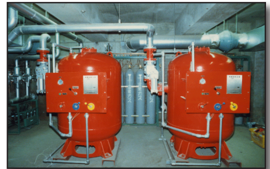
Figure 11-50 Dry Chemical System Storage Tanks
