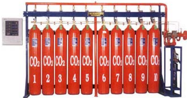
Figure 11-49 Carbon Dioxide System Storage Tanks
