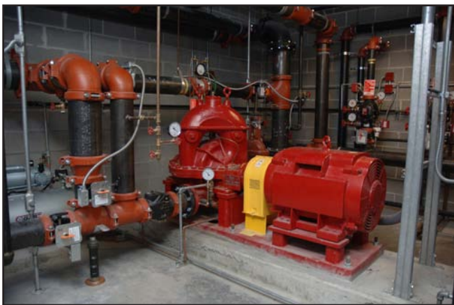
Figure 11-42 Fire Protection System Pump
