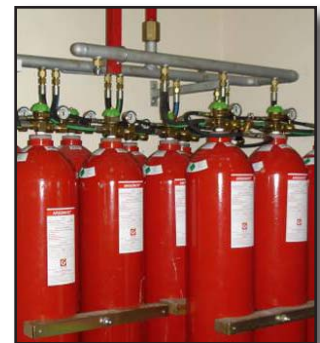
Figure 11-48 Halon Storage System
